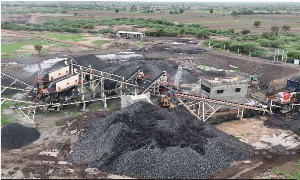
250 TPH - 3 STAGE C&S PLANT WITH WASHING SYSTEM
