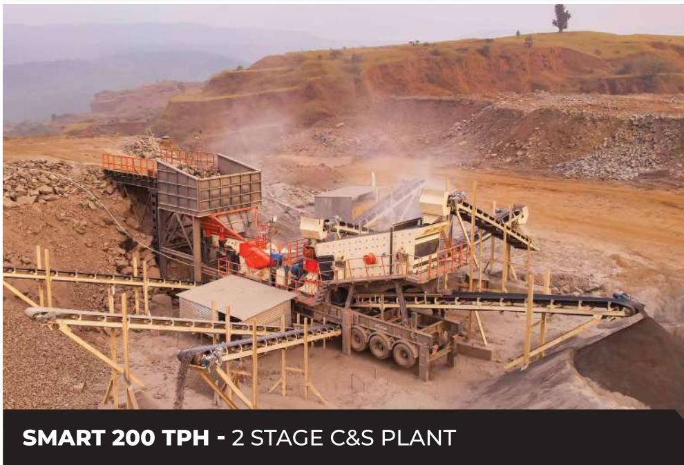
350 TPH - 3 STAGE C&S PLANT WITH WASHING SYSTEM
